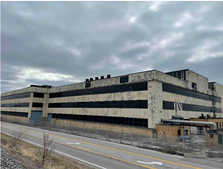
Photograph 11: View of potential bat habitat (abandoned building with broken windows and other outside connections) within the Northern Tract site
